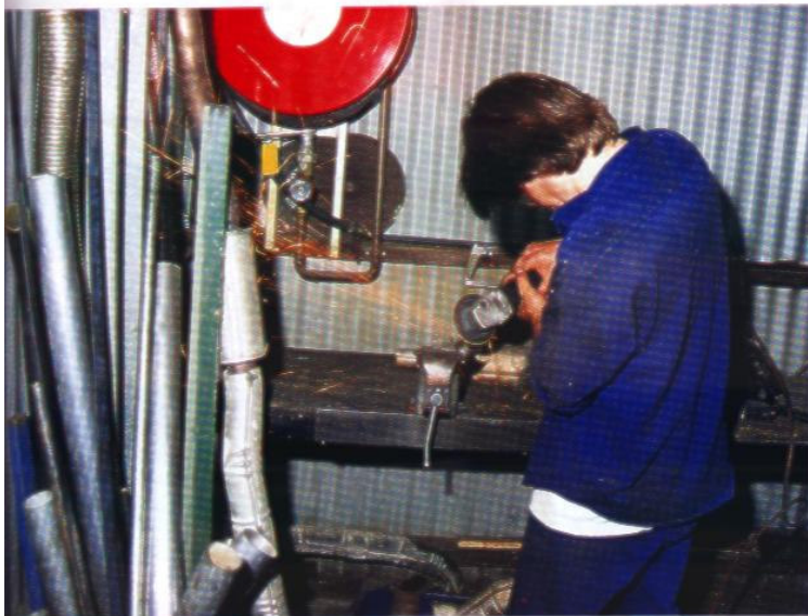
Fabricating the turbo pipework is a labour intensive job, adding to the cost of the exercise
